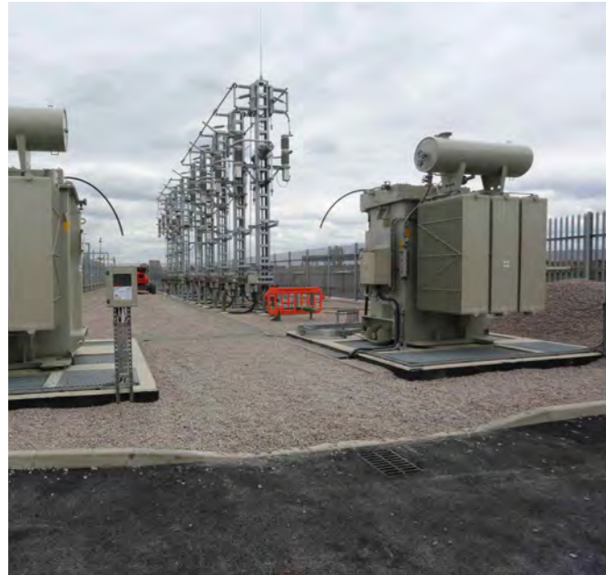
Typical appearance of Auto-transformer Station ©RailTechnologyMagazine
