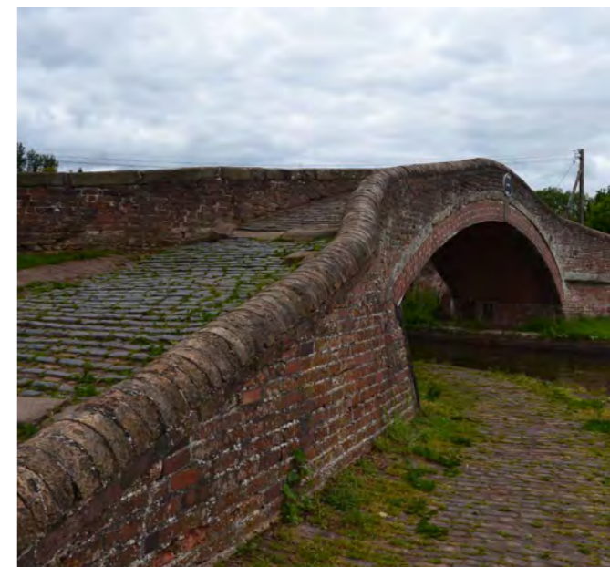
Haywood Bridge Scheduled Monument, with surviving historic materials to the bridge and surfaces
